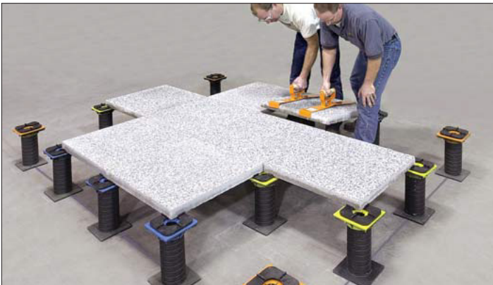
11- Run two or three rows of pavers down the middle of the deck in both directions. Keep pavers straight with laser.
